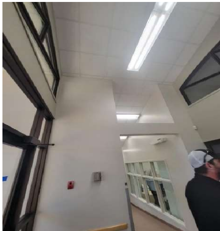
Acoustic Ceiling Treatment (Susp. T-Bar)
