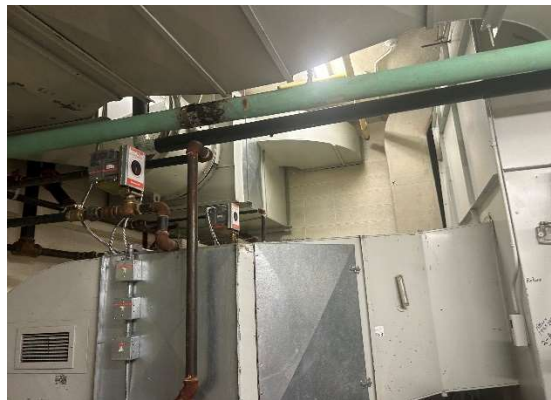
Air Handling Unit – Mechanical Room
