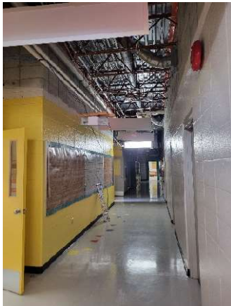
Ductwork Distribution in Hallways
