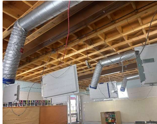
Typical Ductwork Distribution in Classroom
