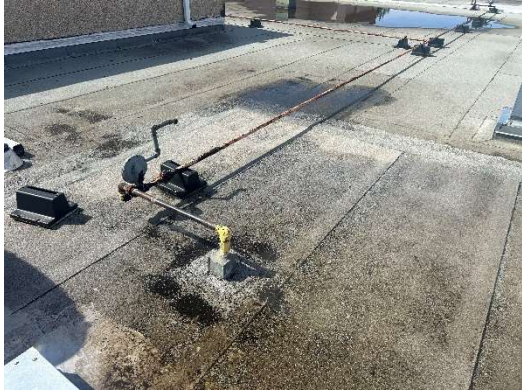
Natural Gas Piping
