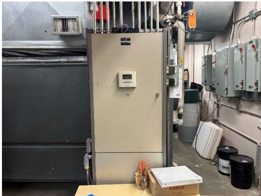
Air Handling Unit – Mechanical Room
