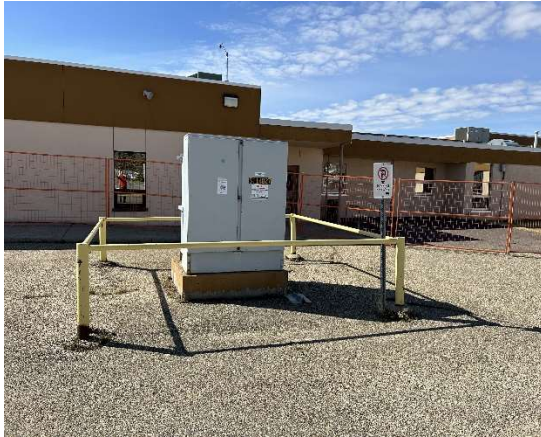
Pad Mounted Transformer
