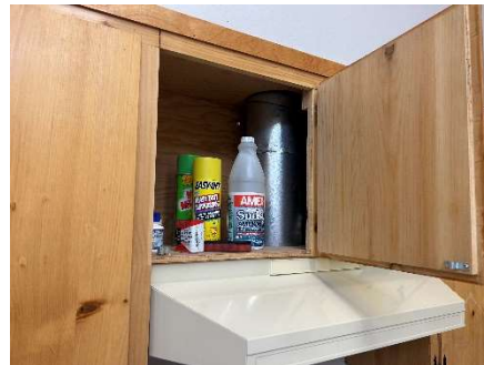
Kitchen Range Hood Fan
