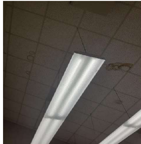
Acoustic Ceiling Treatment (Susp. T-Bar)
