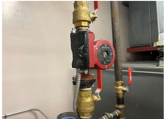
Boiler Circulation Pump – Mechanical Room
