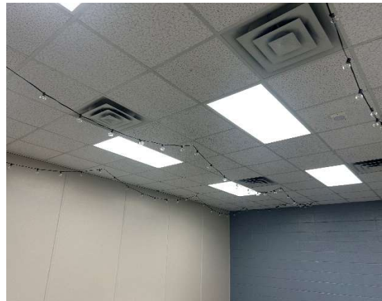
Typical Diffusers Serving Classrooms
