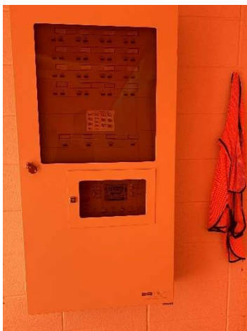
Fire Alarm Panel
