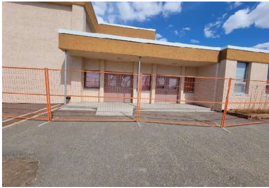
Limited concrete stairs around the site.
