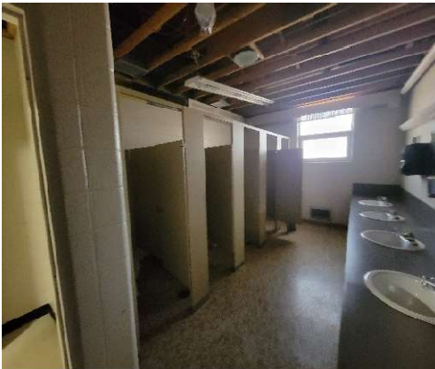
Fabricated Compartments (Toilets/Showers)
