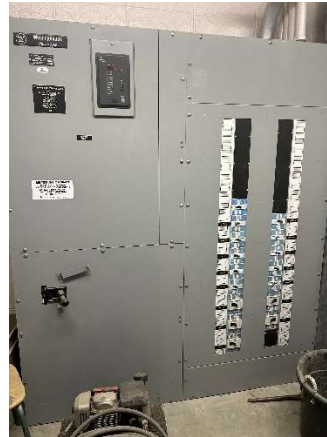
Main Distribution Switchgear
