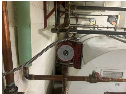
Domestic Hot Water Recirculation Pump
