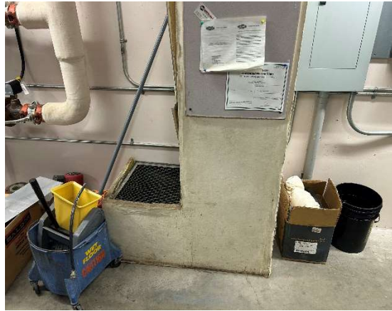
Combustion Air Duct
