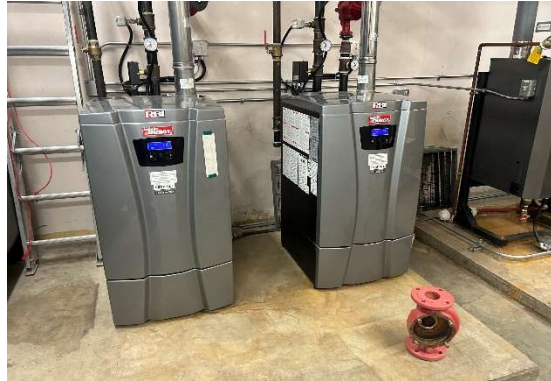
Boilers – Mechanical Room
