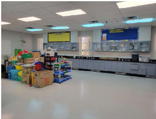
Acoustic Ceiling Treatment (Susp. T-Bar)
