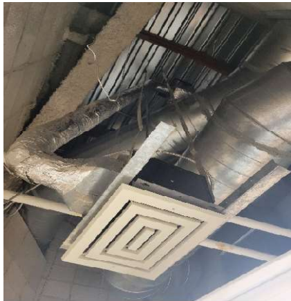
Ceiling Mounted Exhaust Fan
