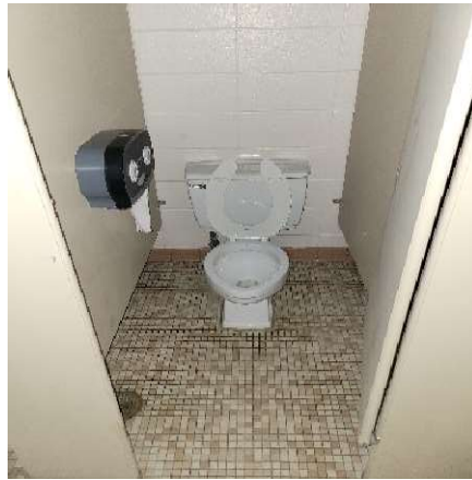
Fabricated Compartments (Toilets/Showers)
