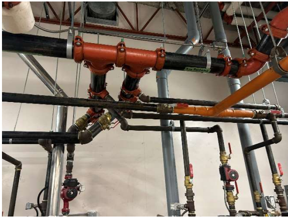
Heating Piping Distribution in Mech. Room
