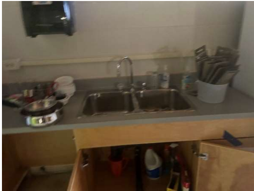
Administration Area Sink
