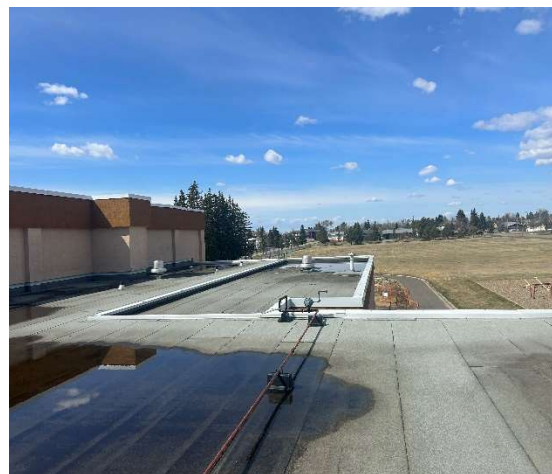
Roof Mounted Exhaust Fans
