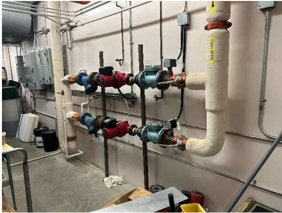
Primary Heating Circulation Pumps
