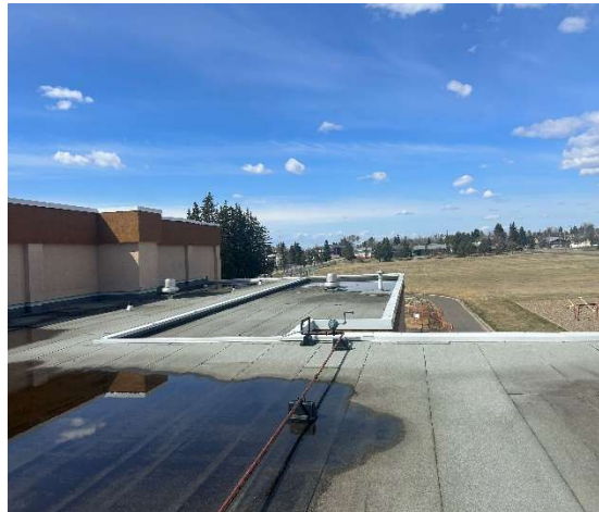
Roof Mounted Exhaust Fans
