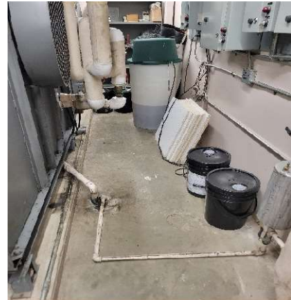
Glycol Make-up System
