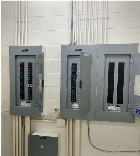
House Branch Circuit Panelboard
