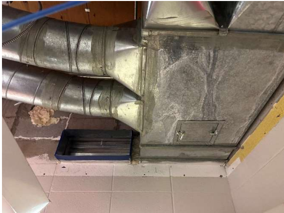
Fire Dampers Serving Duct Penetration
