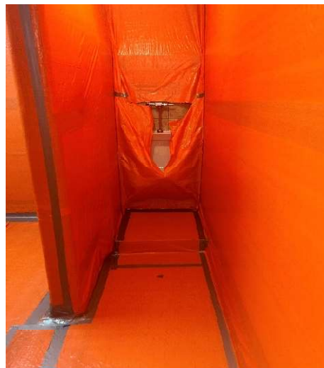
Urinal in Gymnasium Changeroom
